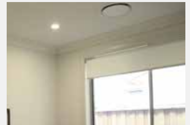
8. SAMSUNG 12KW DUCTED AIR CONDITIONING
