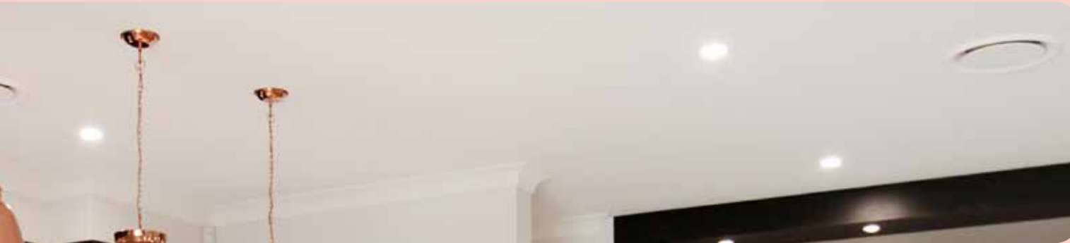
Dakin 12.5kW Inverter Air Conditioner with a Dakin Zone Controller to keep you cool
