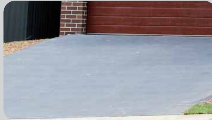
And as always, your driveway is included standard as part of your new home
